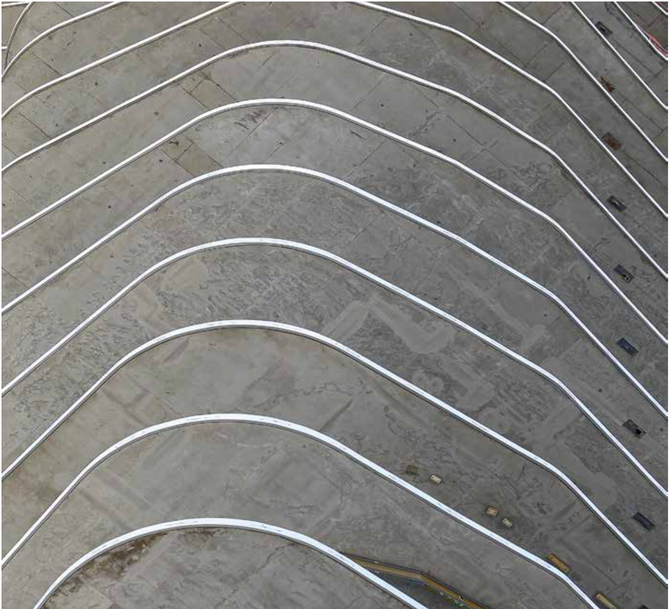
Multi-story high-rise undulated slab edge completed through constructable design practice. Image courtesy of Ceko Concrete Construction.
