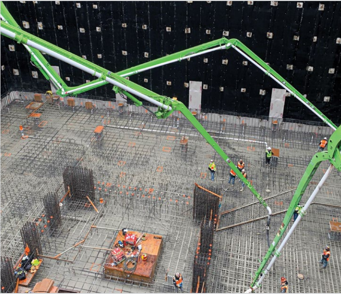
Mat foundation pour six levels below street; The Ayer included six levels of subterranean parking and three levels of parking above grade.
